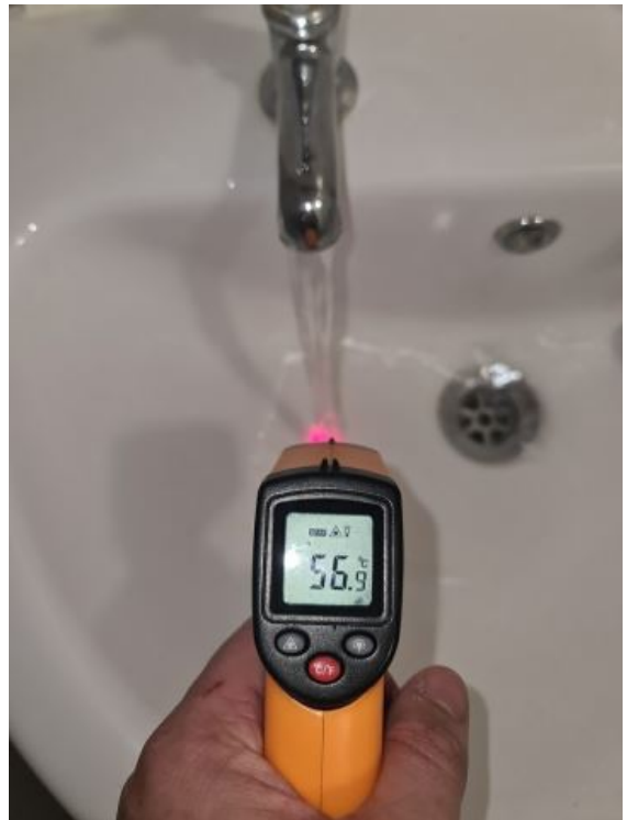
Image 4: Hot Water System
