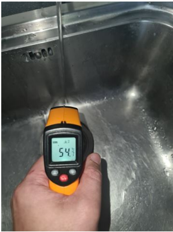
Image 5: Hot Water System
