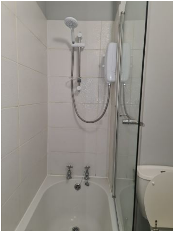
Image 6: Deadlegs and Hoses
