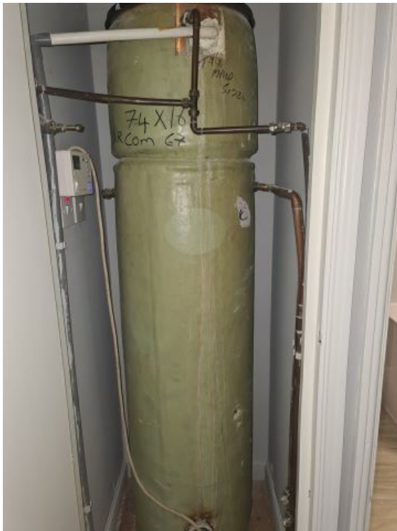
Image 3: Hot Water System
