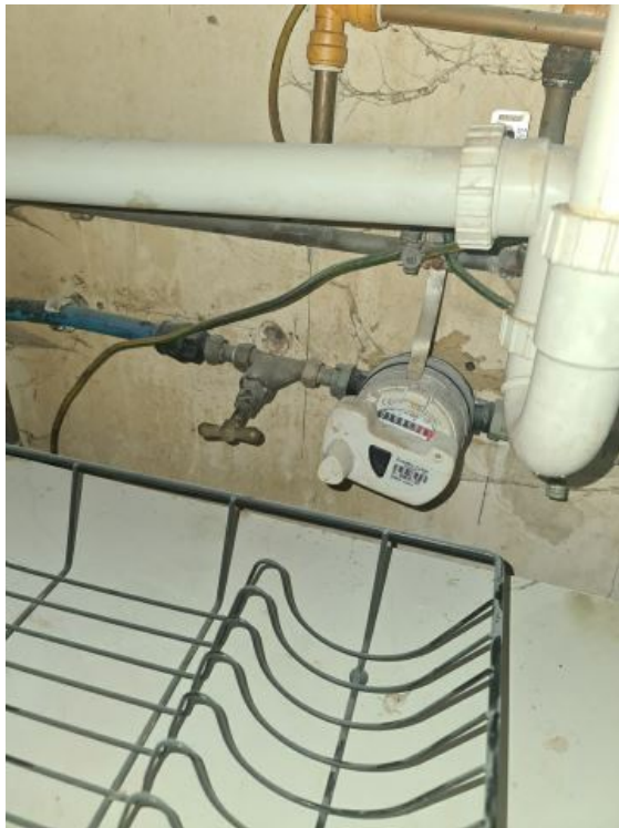
Image 0: Cold Water System
